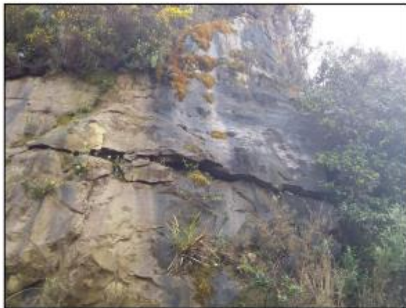
Figure 1 Requires regular monitoring for possible movement
