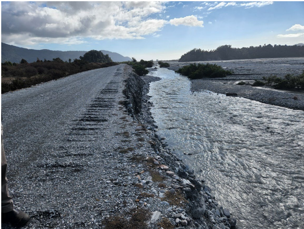
Image 4: Looking downstream towards Rata Knoll and the Waiho Loop. There is potential for more erosion to occur on this bank. The longer it is left untreated the more it is going to costs to repair and armour the area.
