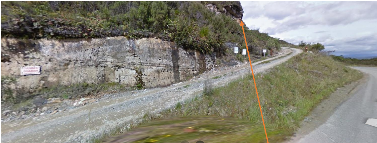
Figure 2 Entrance in 2009 when the site was in use. The area of rock identified as a risk is shown above. This photograph does not show the recent roading improvements that have been made to Roa Road.
