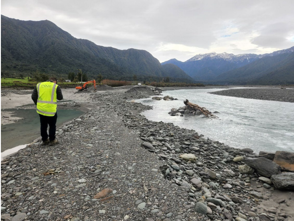
Image 3: Looking upstream along the damaged stopbank
